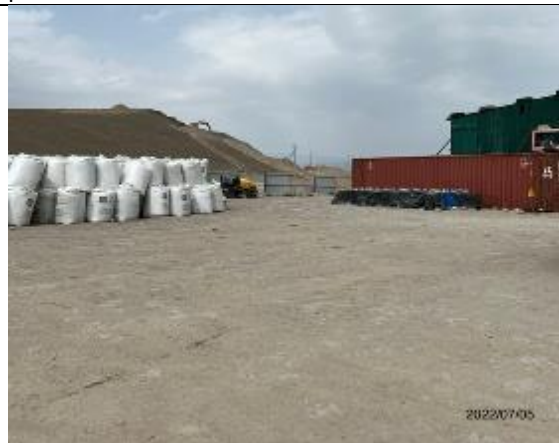
Photos 70. Sanitary condition of the territory of the production base is satisfactory
