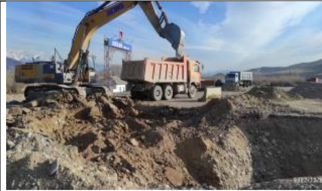
Photos 22. Digging a pit for the construction of an underpass at km 86+325 RHS
