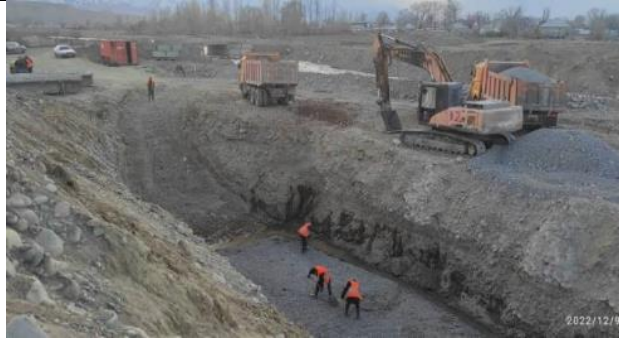
Photos 34. Construction of the bridge at km 65+410. Construction of the foundation for the bridge piers
