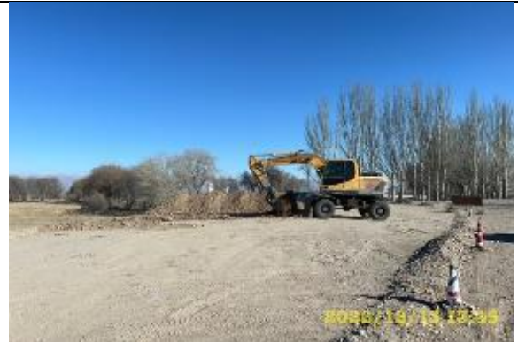
Photos 23 Trenching and excavation at km 0+153 (new circle) for a new culvert
