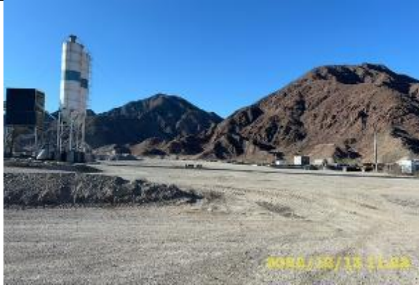
Photos 56. Lot 1. Production base. PRODUCTION FACILITY. Sanitary condition of the territory of the industrial base is satisfactory.
