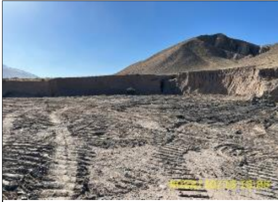
Photos 80. Leveling of the old asphalt dump located on the right side of the road at km. 89+093
