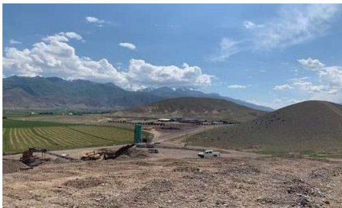
Lot 2 facility area with the rock crushing plant at the foreground and the Contractor's camp at background.
