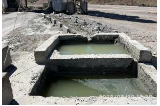
Photos 57. 3-chamber primary wastewater treatment tank BSU Lot 1.
